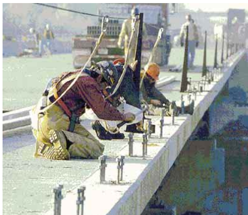
MetaMax® HRM used in high-performance concrete on dual four-lane bridges carrying I-87 over the Hudson River.
