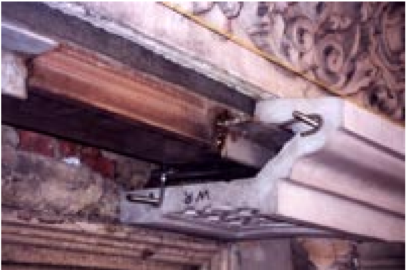
Due to the landmark status of the building, the team tried to replace deteriorated facade elements with matching terra cotta as far as possible.
