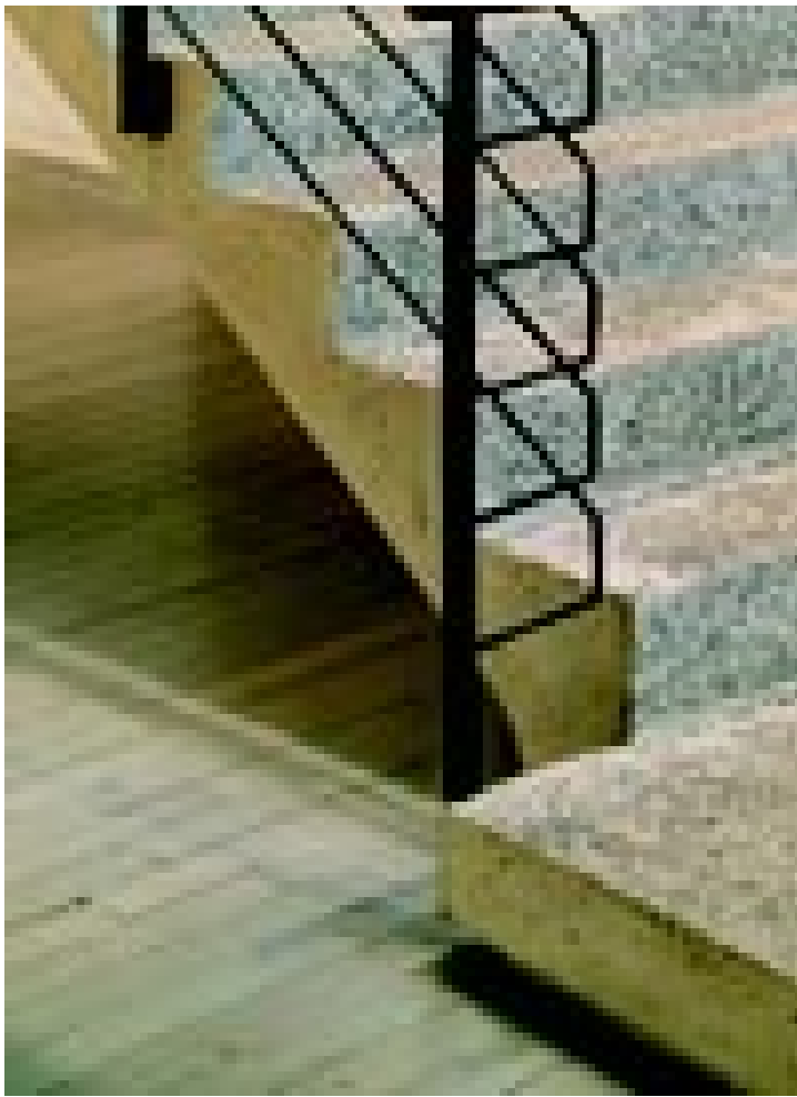
Built in one continuous pour, the flight's 24 inches thickness at the bottom sweeps to a mere four inches at the top and is shaped to resemble the keel of a boat (Image © Peter Aaron/Esto).
